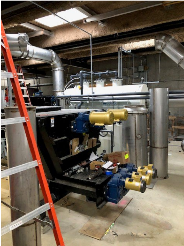
Packed Tower & Hopper in Upper level
