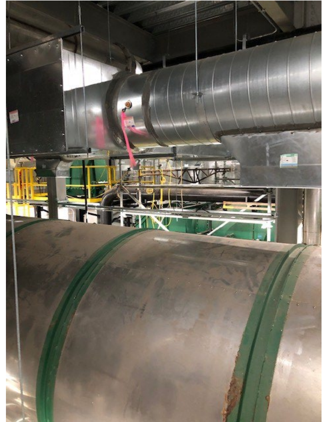
Gasification & HVAC Ducting in Lower level.
